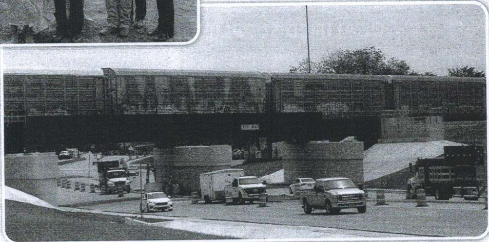
The railroad bridge had to be rebuilt as part of this expansion project.
